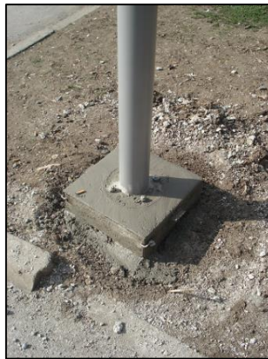
Figure 5.2-2. Street lamp with concrete ( beton ) poured on its ground, 04.02.2009
